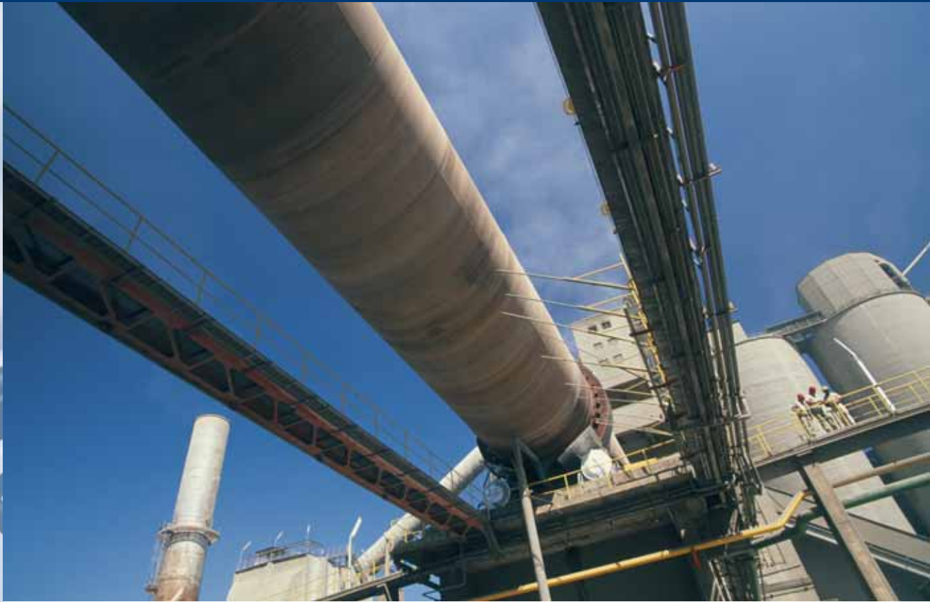
Rotary Kiln with DC-Motors
